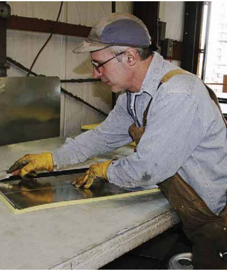
A sheet metal worker cuts polyimide foam duct liner for the Daniel J. Evans Library project. His cutting template is the same piece of sheet steel the liner will be attached to in the duct.
